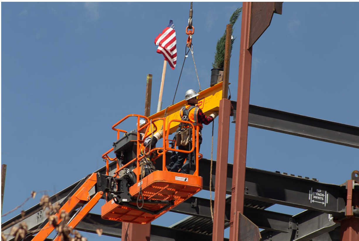
The last steel beam is set into the frame of the new building, which is scheduled to open in spring 2020.
