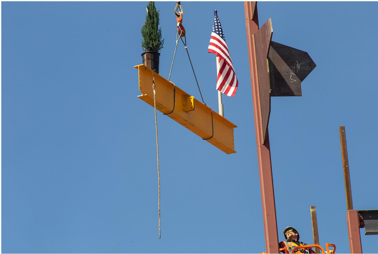
Last steel beam for the new Contra Costa County administrative building is hoisted in the air.
