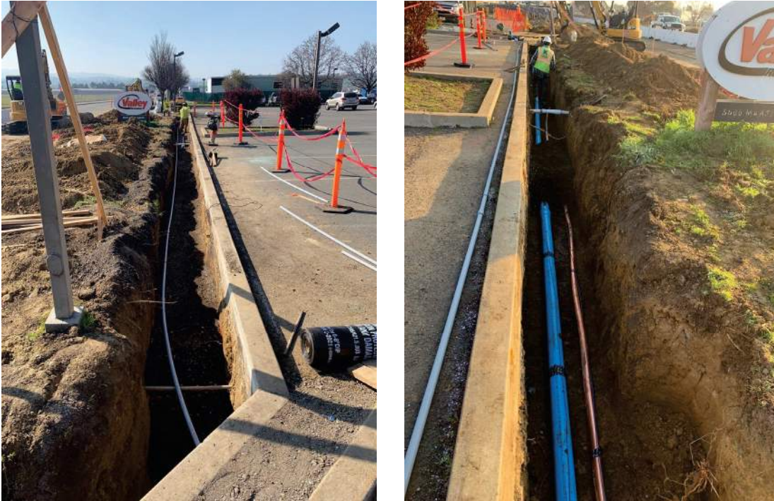
Figure 4 – CCWD Waterline – Tamper Switch Conduit + 2” and 4” Water Service Lines
