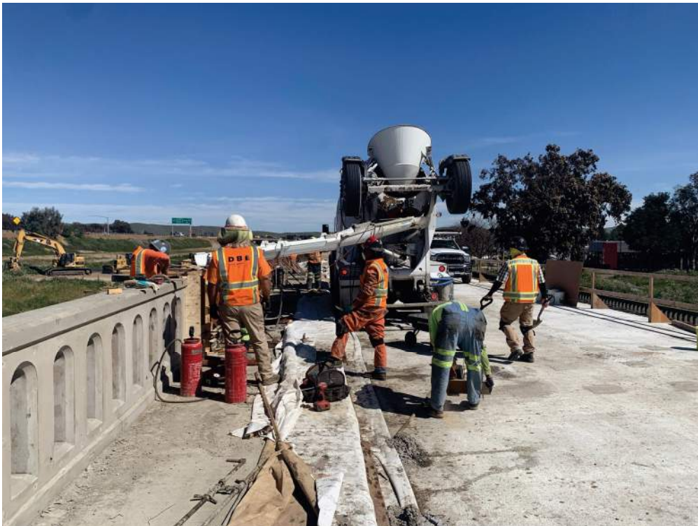
Figure 4 – Bridge Concrete Railing
