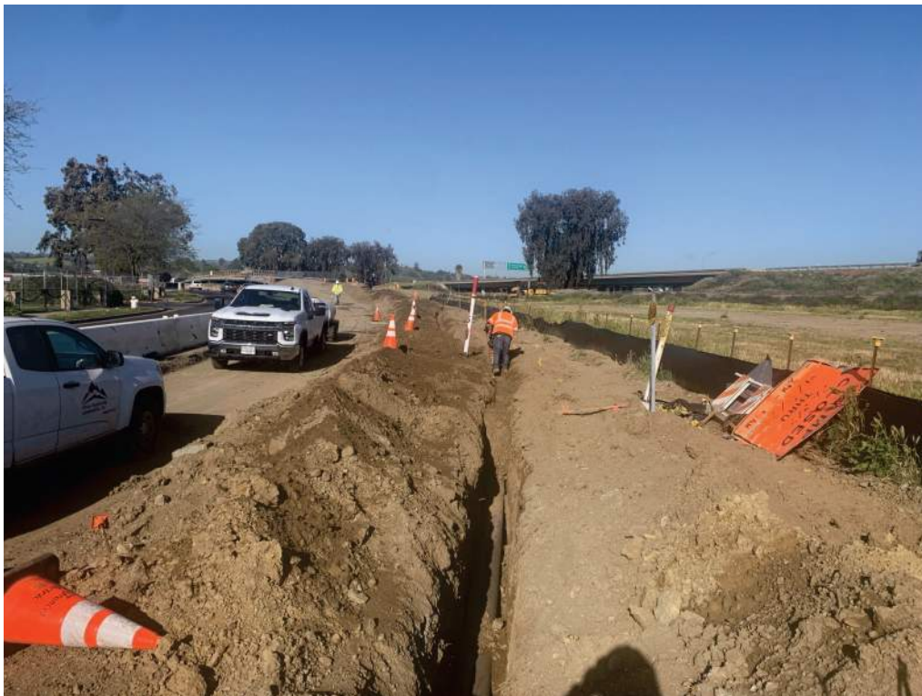
Figure 3 – AT&T Conduits (Eastside)
