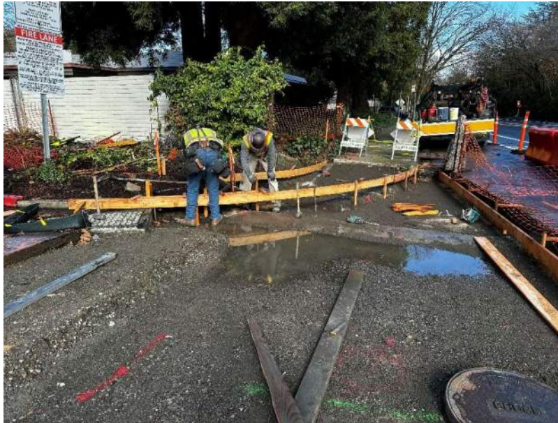
Figure 1. Crews placing formwork for the driveway and curb ramps at the Jackson Intersection
