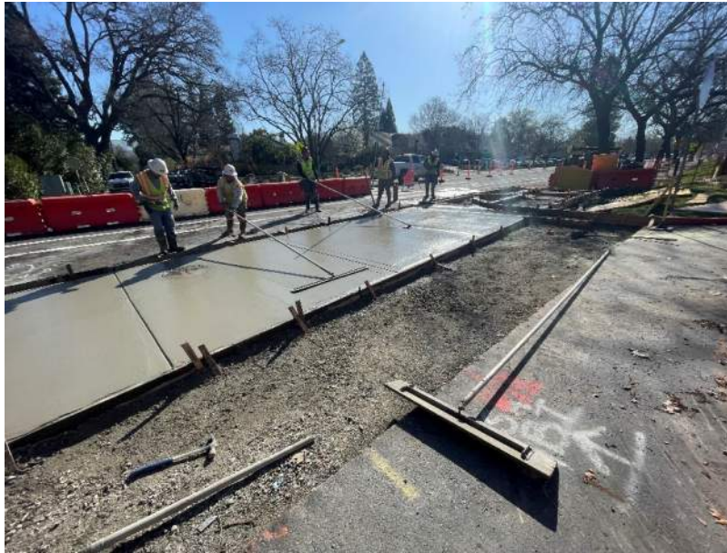
Figure 1. Crews finishing concrete for the driveway and curb ramps at the Jackson Intersection
