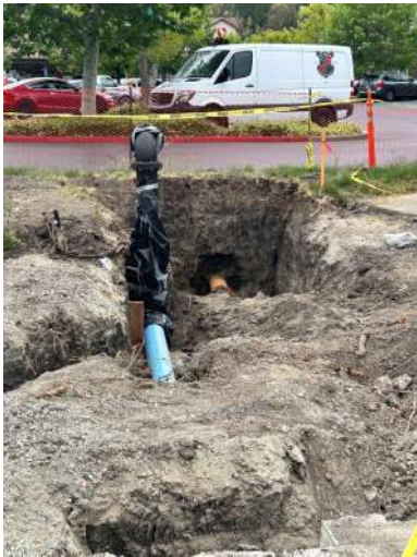
Figure 1. - Fire Supply Installation
