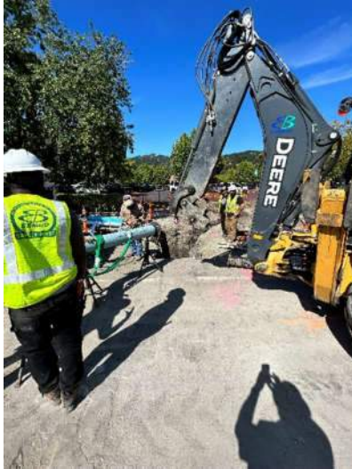
Figure 1. - EMBUD Fire Water Connection
