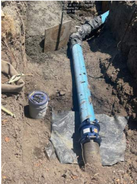
Figure 1. - Fire Water Installation
