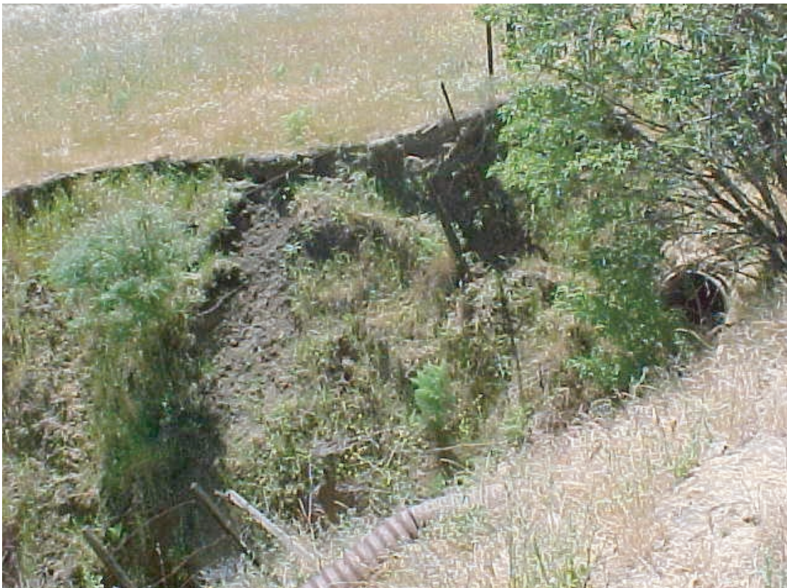
Channel erosion caused by poorly maintained culvert in Upper Kirker Creek
